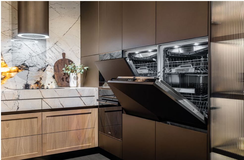
Two full-size dishwashers with lighting and an automatic opening system have been designed and installed at an ergonomic height.
